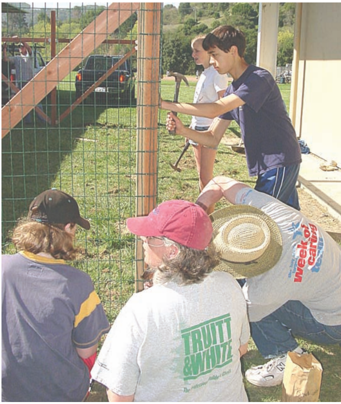
8th graders Leanne Woehleke and Connor Ludwig nail the fence to the posts while Shelby Watts (6th grade), Claire Curtin and Steve Woehleke lay chicken wire to discourage unwanted guests
