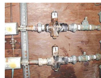
Two valves of the HVAC system similar to the one that failed in April 2007
