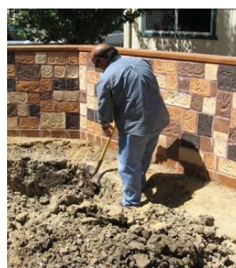
Excavating the wall stallion in another location at an as yet undetermined date.
