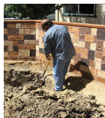
Excavating the wall stalling in another location at an as yet undetermined date.
