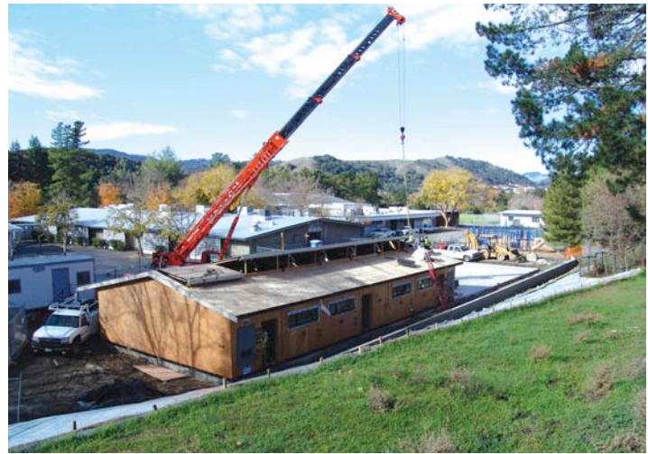
J.D. Arrighi & Mike Snow, Meehleis Modular Building Inc., set a roof piece on Saturday morning
