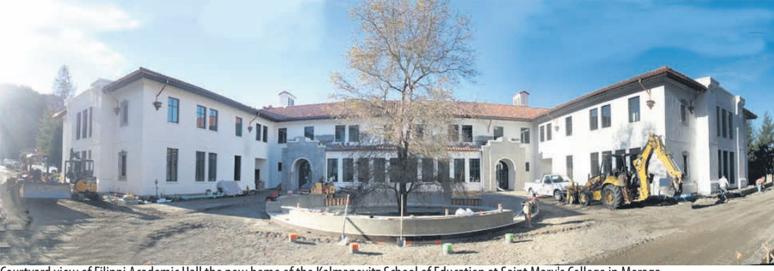
Courtyard view of Filippi Academic Hall the new home of the Kalmanovitz School of Education at Saint Mary's College in Moraga.
