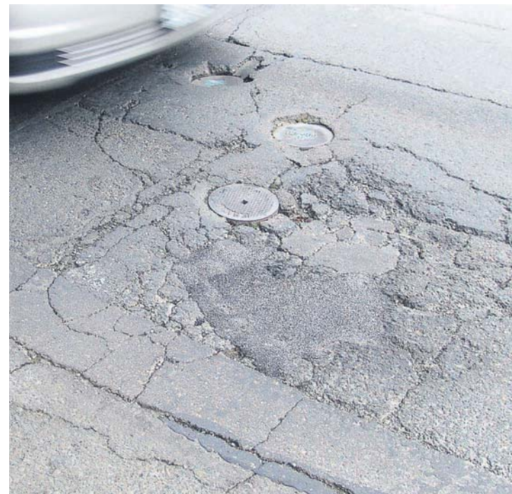
Rough road conditions on Moraga Way Photo Andy Scheck
