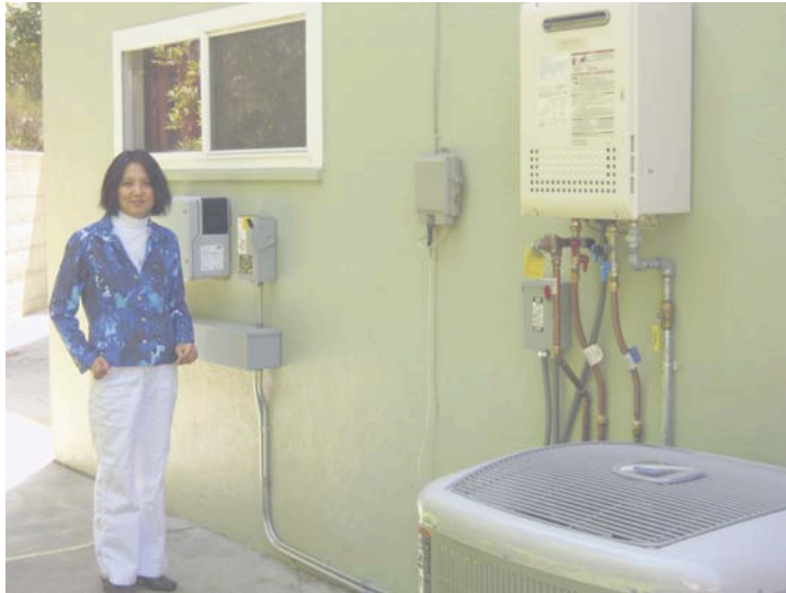
Joann Tan checking the solar meter and the tank-less water heater in her Lafayette home
