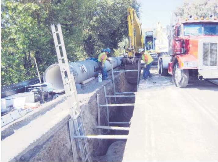
7-ton pipes are set in a 10 foot deep trench Photo Sophie Braccini
