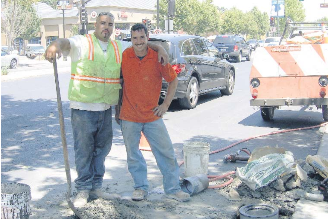
Hard-working employees of St. Francis Electric, a subcontractor of Top Grade Construction Photo Cathy Tyson
