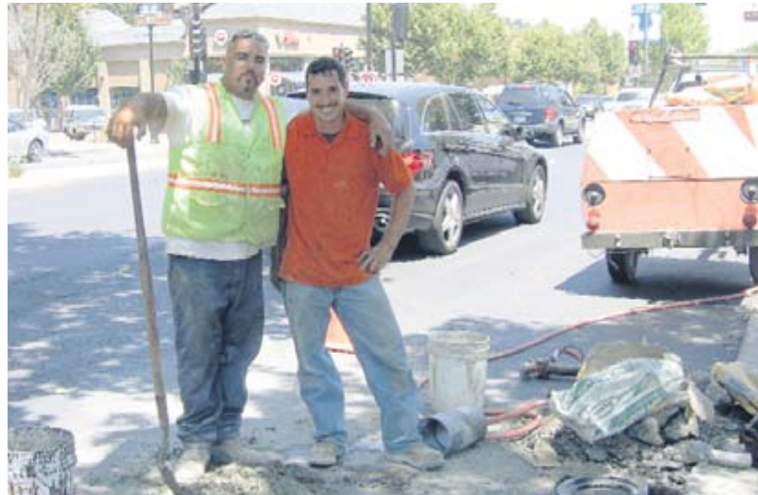
Hard-working employees of St. Francis Electric, a subcontractor of Top Grade Construction Photo Cathy Tyson
