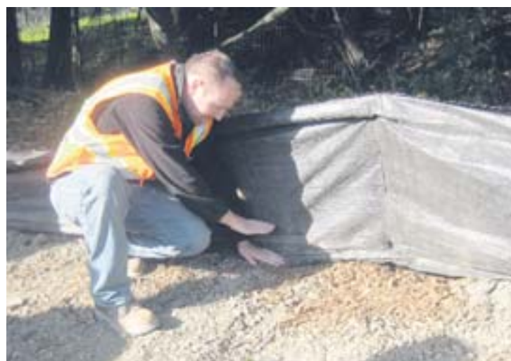
Kevin Fitzpatrick explains how the protective fence works
