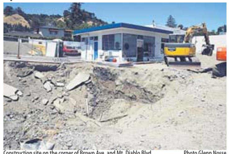
Construction site on the corner of Brown Ave. and Mt. Diablo Blvd. Photo Glenn Nosse
