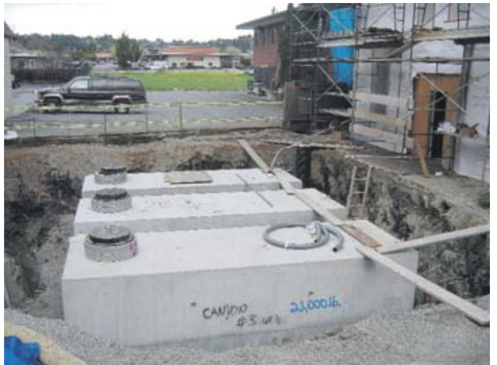
Concrete tanks were buried by "The Barn" at the time of its renovation.
