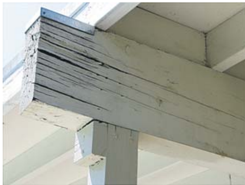
Dry rot on a roof beam
