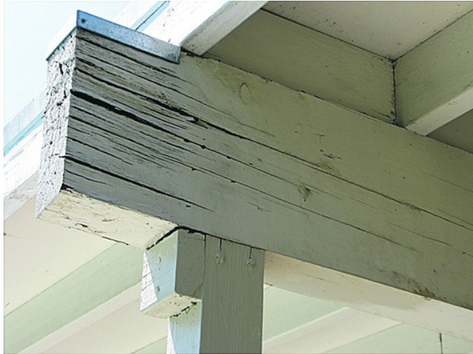
Dry rot on a roof beam
