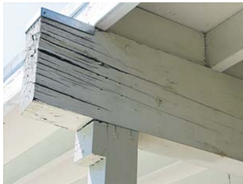
Dry rot on a roof beam
