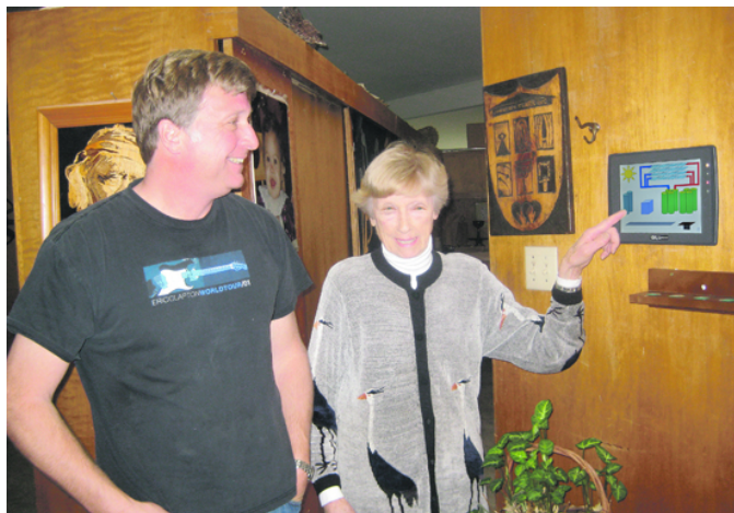
Louise Clark (R) and son Charles Clark next to the control panel for their geothermal system Photo Sophie Braccini
