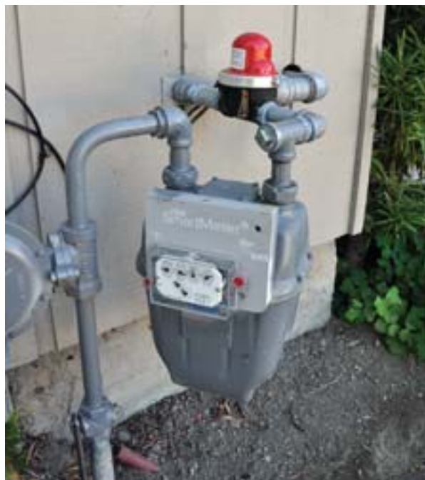
Gas meter with seismic valve
