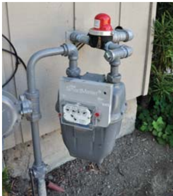
Gas meter with seismic valve
