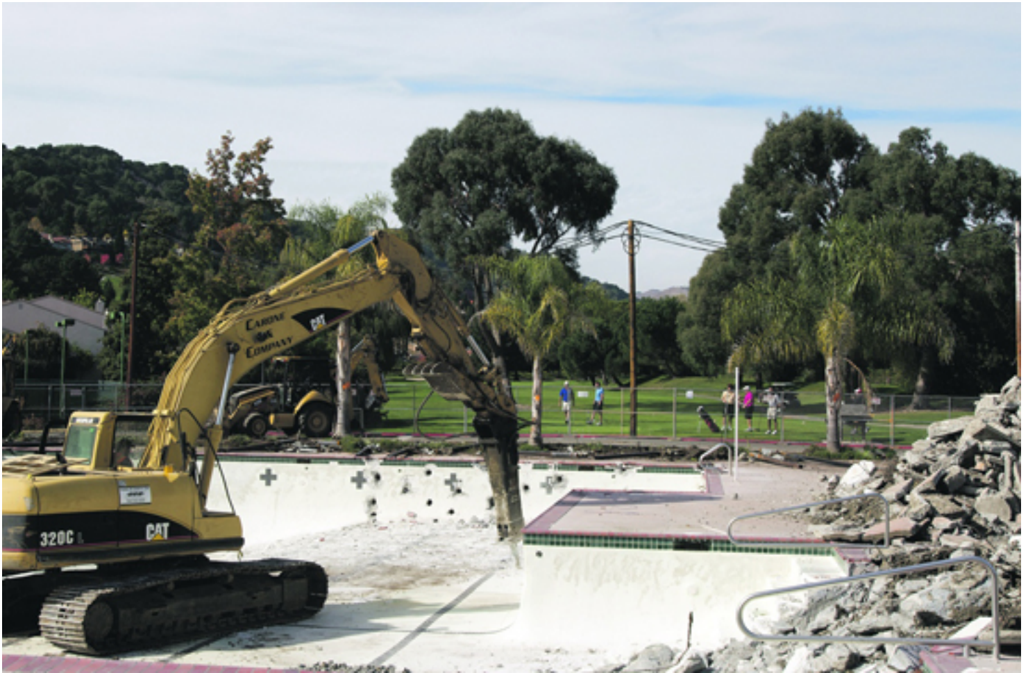
Old concrete will be recycled and reused at the site Photo Doug Kohen
