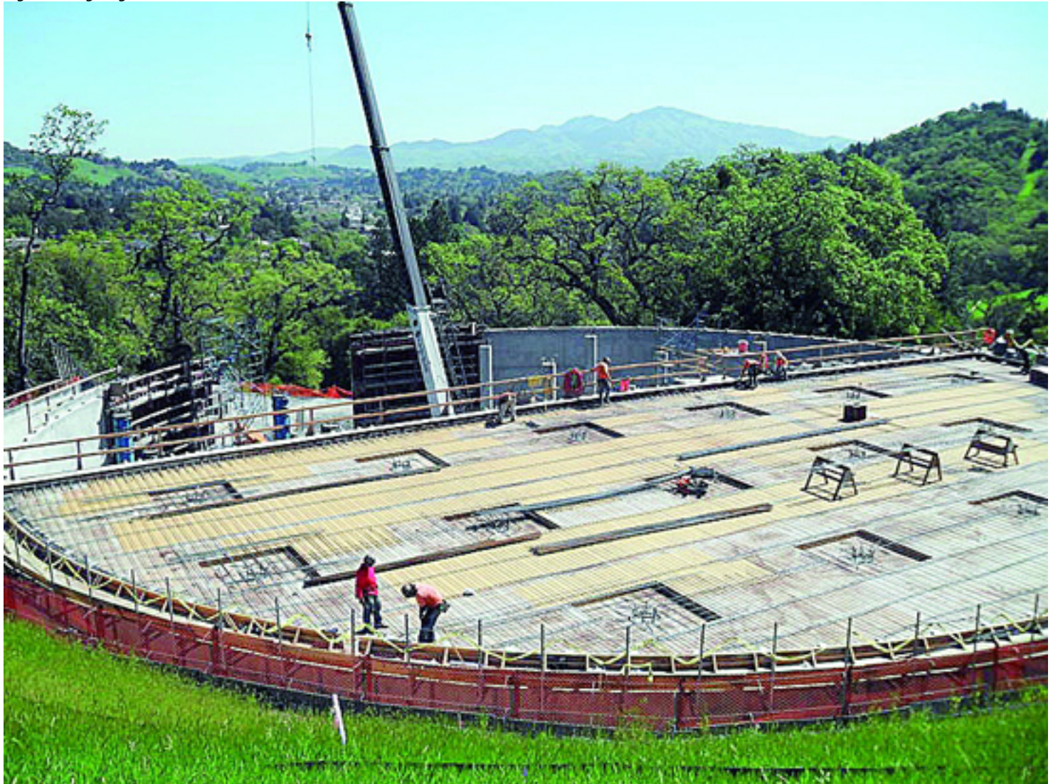
Crews working on the partially completed Highland Reservoir last week. Photo C. Tyson
