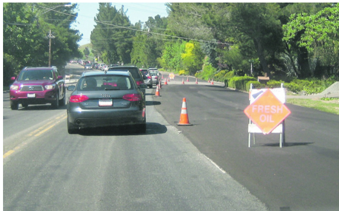
Long lines of cars as the road is repaved Photo Sophie Braccini
