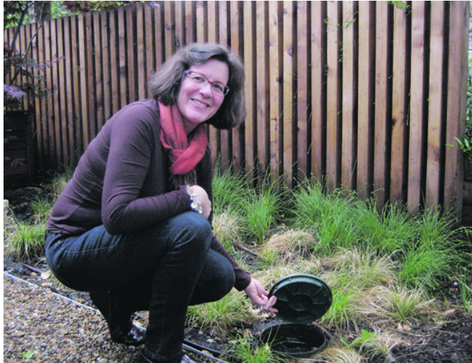
Gwenn Lennox shows the entrance to the gray-water collection tank. Photo Sophie Braccini
