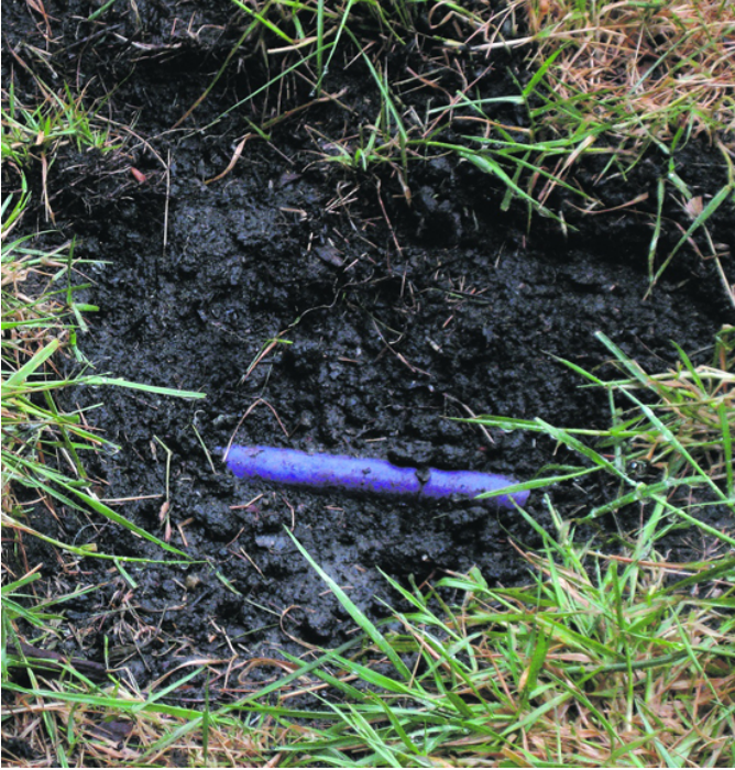
Purple drip lines containing gray-water irrigate the lawn.
