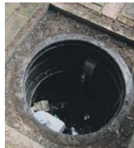
Access to the rainwater containers under the patio
