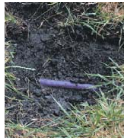
Purple drip lines containing gray-water irrigate the lawn.
