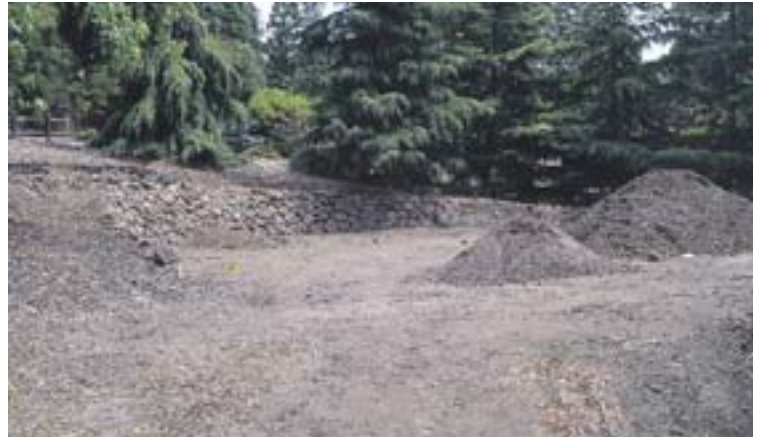
Ground has been broken for an outdoor labyrinth at St. Stephen's Episcopal Church, Orinda.
