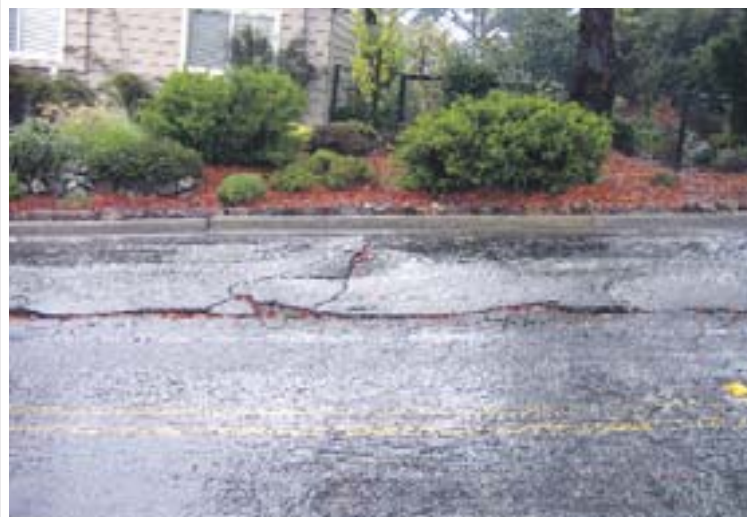
Urgent issues such as this one on Zander Drive receive priority attention from Orinda's Public Works and Engineering Department.
