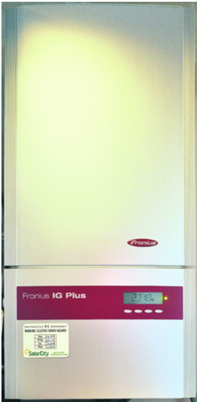
The indoor inverter is mounted on a garage wall
