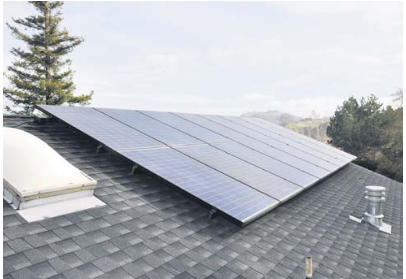
The biggest of our three solar panel arrays holds 16 of the 32 panels.
