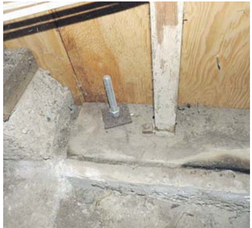
Retrofit anchor bolt with plate washer (on left) shown next to original anchor bolt and small washer.
