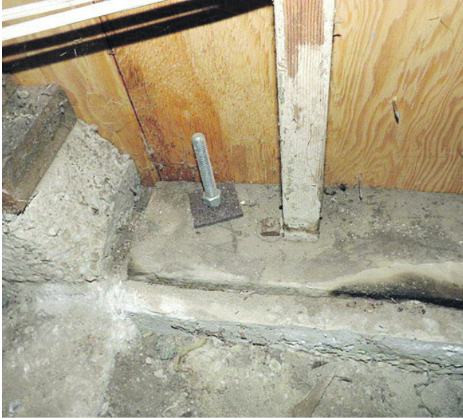
Retrofit anchor bolt with plate washer (on left) shown next to original anchor bolt and small washer.
