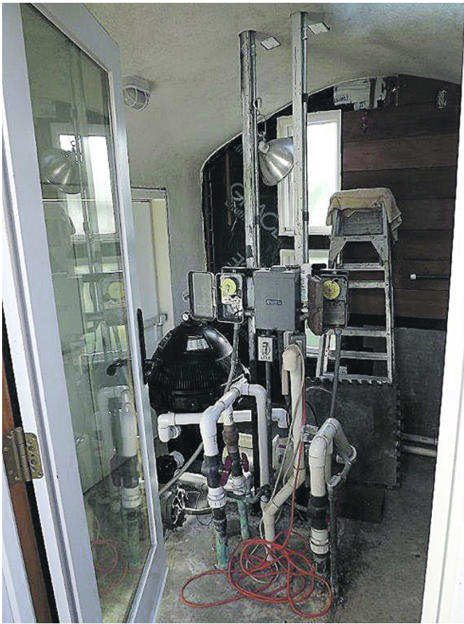
The Walters' pump house Photo Cathy Dausman
