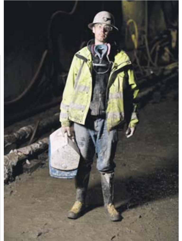
Selected images from "Tunnel Vision," an award-winning series of photographs capturing the construction of the new fourth bore for the Caldecott Tunnel, are also currently on display at the Orinda Library Art Gallery this month. Drivers felt a glimmer of hope for easier commutes late last year with the news that eastern and western tunneling operations had finally connected. The new $402.1 million bore – "one of the largest recipients of Recovery Act funding in the nation," according to regional transportation officials – is expected to open to traffic by late 2013.
