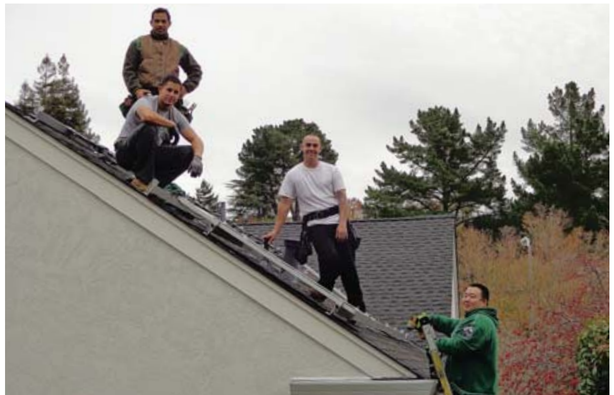
A local solar company installs, monitors, and finances residential and commercial energy systems. They are licensed to install, maintain and repair solar energy systems and for heating, ventilating and air conditioning. Some of the crew are pictured installing panels on a home in Moraga. Photos Cathy Tyson
