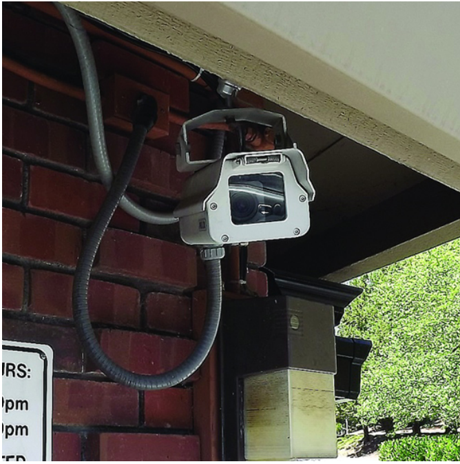
Typical surveillance camera Photo Cathy Dausman
