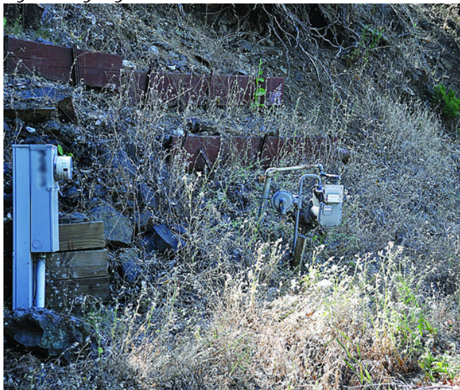
Gas meters like this one in Orinda could qualify for PG&E's Meter Protection Program. Photo Andy Scheck
