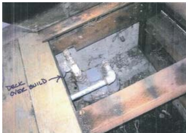
This over build gas meter in Lafayette qualified for PG&E's Meter Protection Program. Photos courtesy Leapfrog Plumbing
