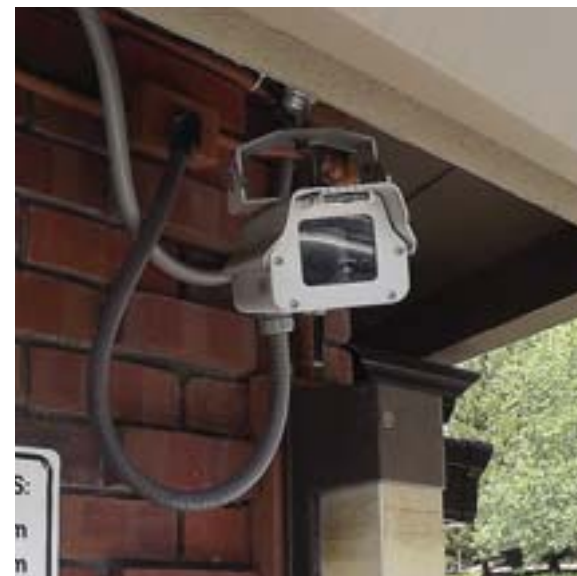
Typical surveillance camera Photo Cathy Dausman
