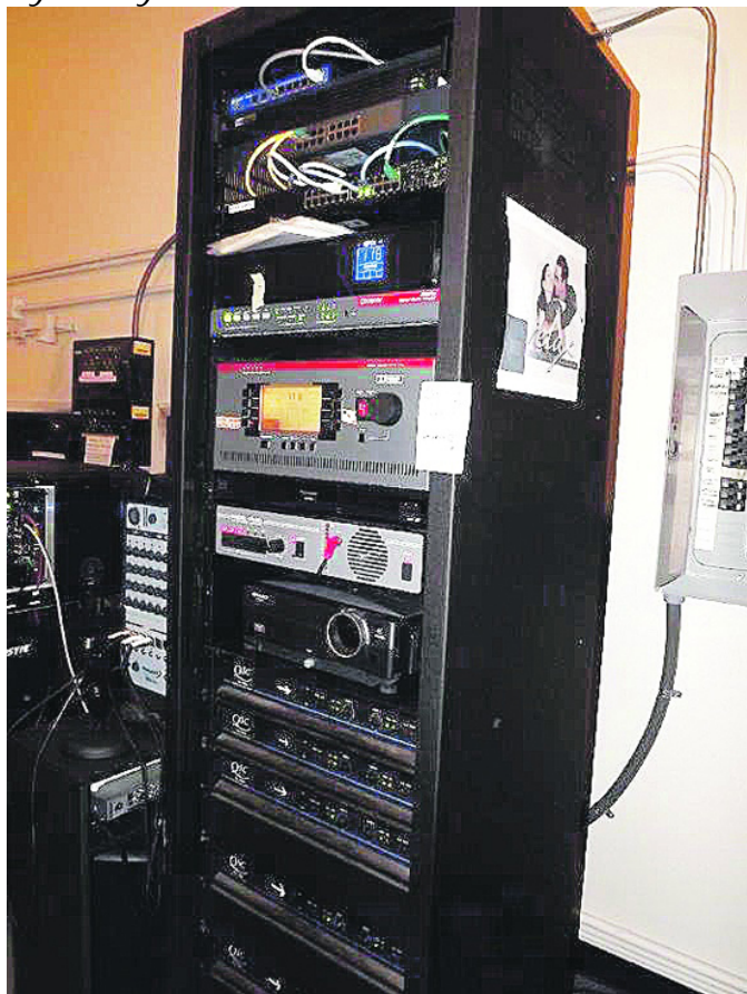
Digital sound equipment at the Rheem. Photos Cathy Dausman
