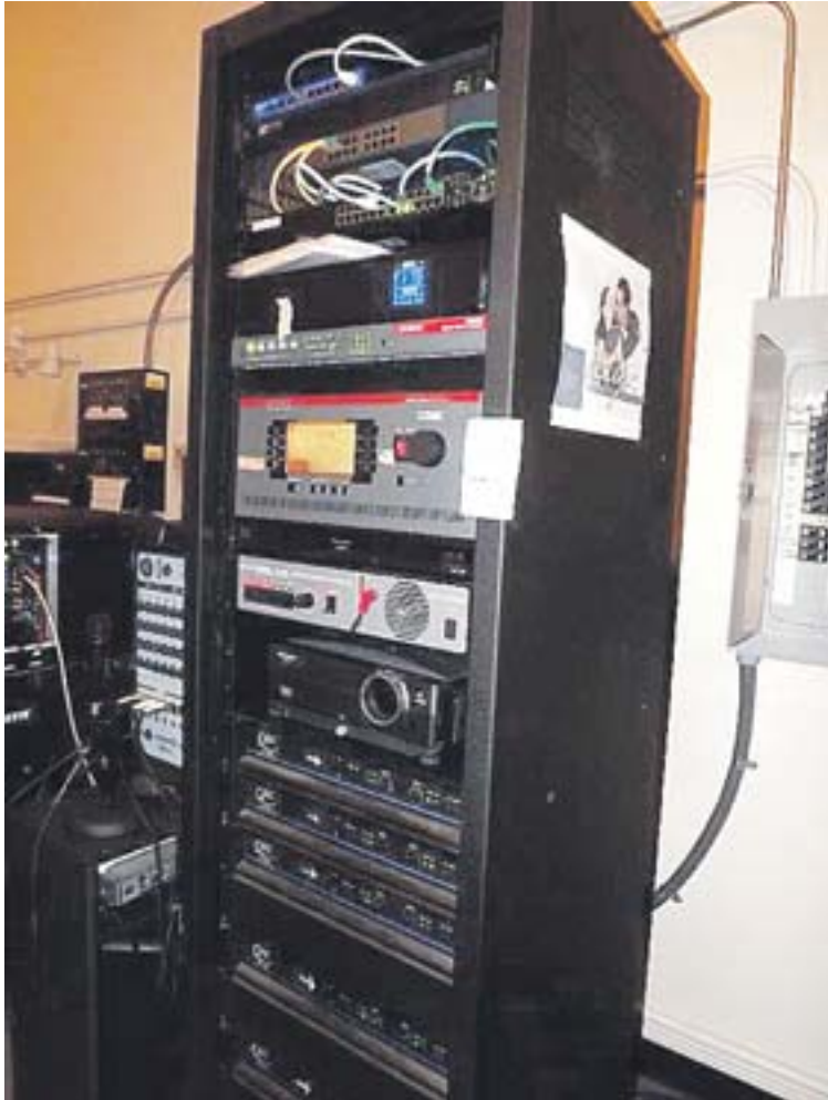
Digital sound equipment at the Rheem.
