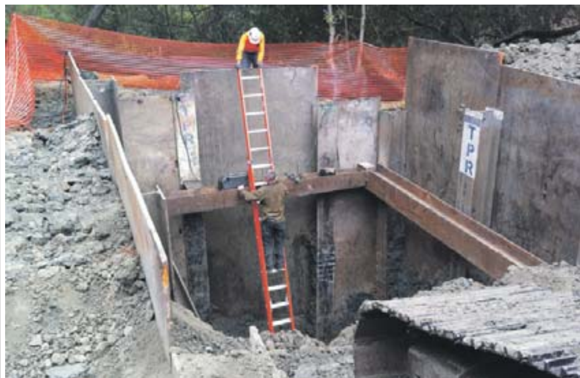
A repair crew is now working its way down to fix a failed drainage system in the Tarabrook neighborhood, which spawned a massive sinkhole last December. A new, sturdier 36-inch concrete drainage pipe will be lowered into this jacking and boring pit—a challenging 25 feet below ground—before workers tunnel and inch the pipe to its final destination. Photo Chuck Swanson
