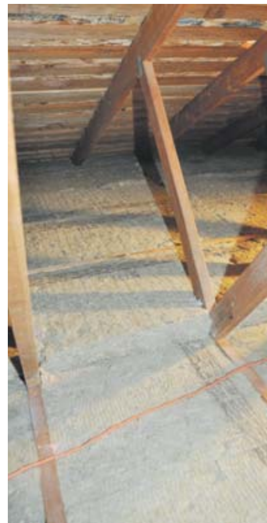
Two perpendicular layers of stone wool insulation batts were easy to install in this Moraga home.
