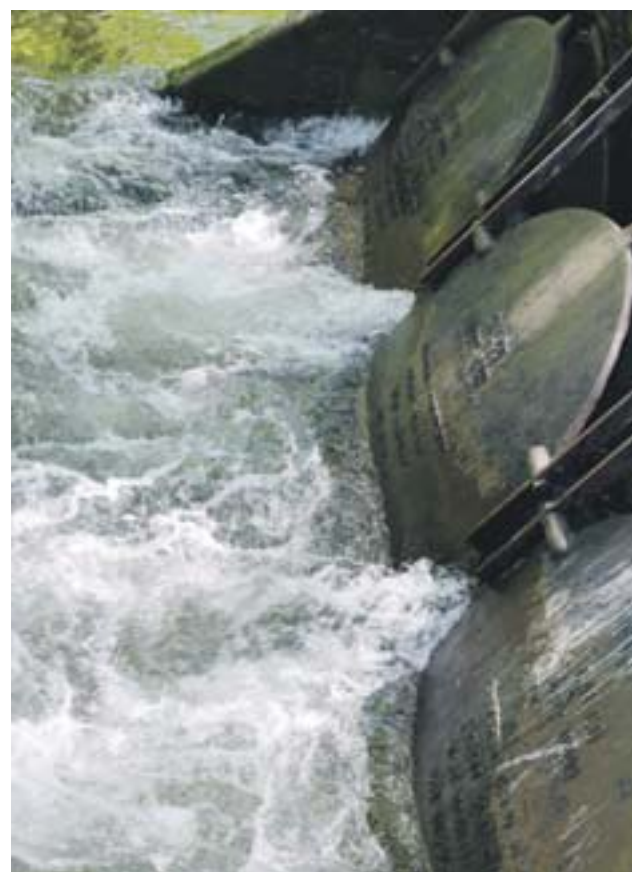
Water traveling 130 miles from the Sacramento River flows through these pipes into the San Pablo Creek at the EBMUD facility off of Manzanita Drive in Orinda. Photo Ohlen Alexander
