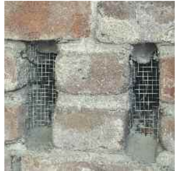
Using 1/8-inch mesh metal screens under eaves or at foundation vents can prevent burning embers from entering a home. Photo Andy Scheck
