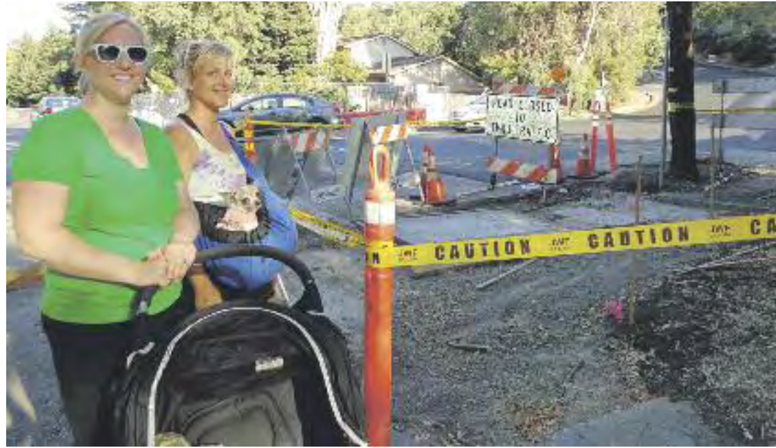
Evening walkers at the intersection of Reliez Station Road and Olympic Boulevard near one of 17 utility structures undergoing work. Photo C. Tyson
