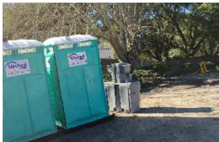
Two unsightly Job Johnnies inhabit this Lost Valley substation.
