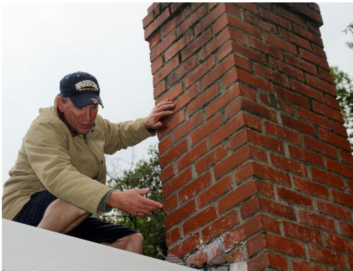
Unseen water can get in between the cracks in the mortar, freeze, and loosen the bricks, making them unstable. Photo Chris Lavin
