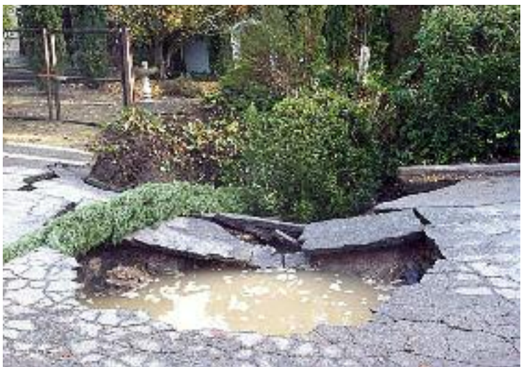
In December 2012, a pipe failure led to the formation of a sinkhole on Tarabrook Drive at Evergreen. Adopting humor in the face of adversity, some Orindans christened the area "Tarabrook Lake" during the worst moments of the emergency. Photo courtesy the city of Orinda
