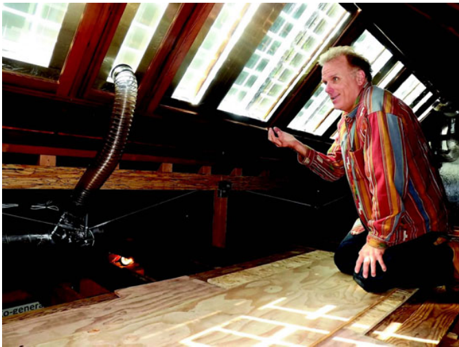
James Wright explains the solar heating system from the attic. Photos Cathy Dausman
