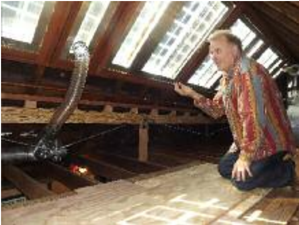
James Wright explains the solar heating system from the attic.
