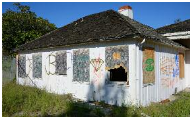
Long a late night party spot for local high schoolers, vandals have inflicted significant damage to the historic Joaquin Moraga Adobe over the years.
