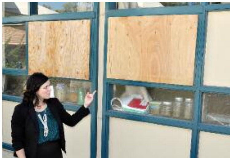
Miramonte High School principal Julie Parks points to boarded windows that were recently broken by vandals at the school.
